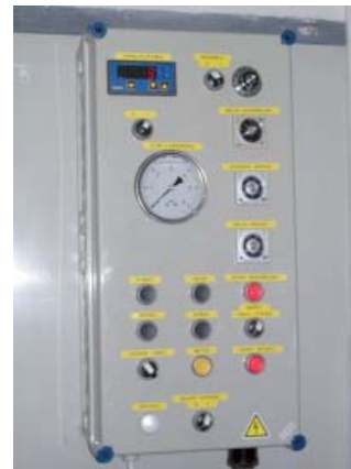
Fig. 8 Operator control unit
