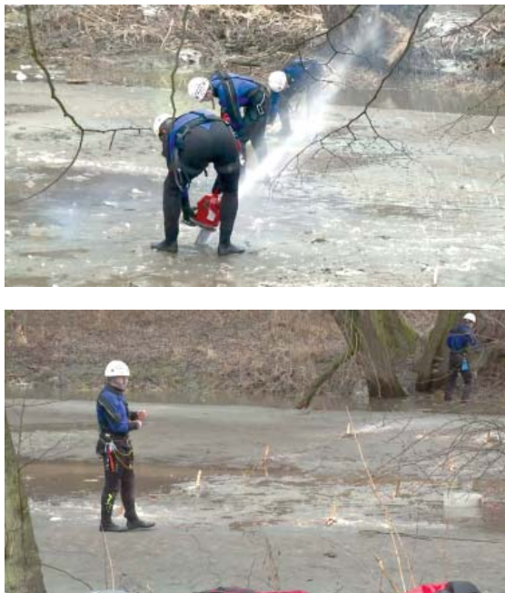
Fig. 5 and 6 The preparation of holes for the placement of charges and the placement of charges beneath the ice surface
