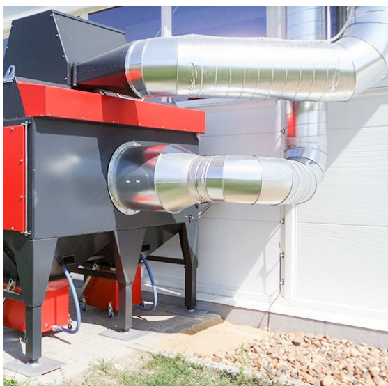
Fig. 2 Filtration and suction equipment (own processing)
