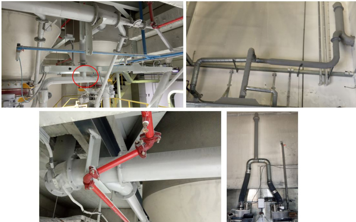
Fig. 5 Air ducts in the workplaces
