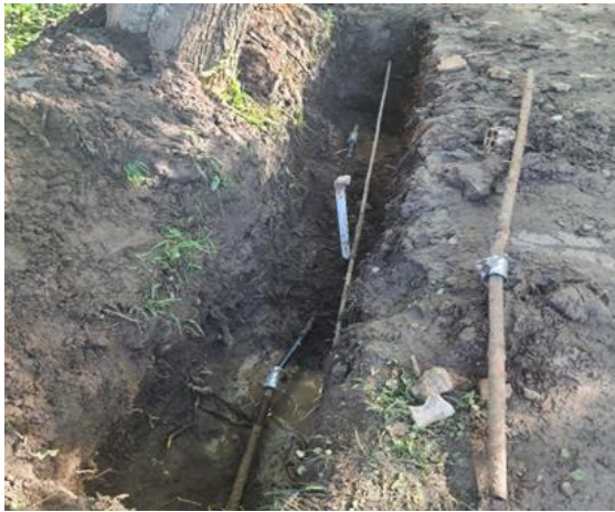
Figure 4. A clamp and fix of a broken drinking water pipe outside of the last author's house in Makhandla, Eastern Cape Province, South Africa. Old pipe and a failed clamp are depicted on the right and the new functional fix (clamp with a new pipe interlink) are shown in dug hole on the left
